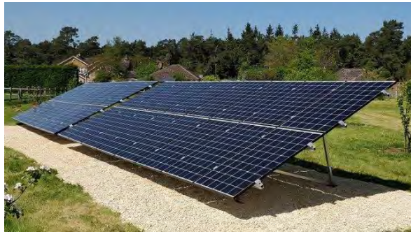
Figure 20: Ground Mounted Solar Panels
