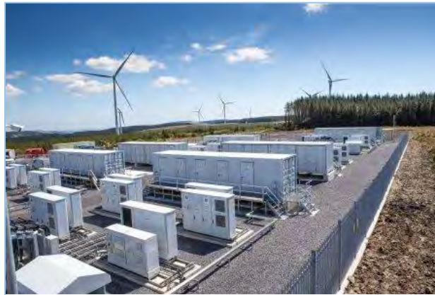
Figure 7: A 22-megawatt BESS facility is co-located at the Pen y Cymoedd wind farm in Wales.
