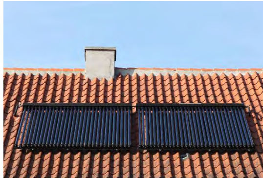
Figure 23: Evacuated Tubes - a bank of glass tubes mounted on roof tiles
