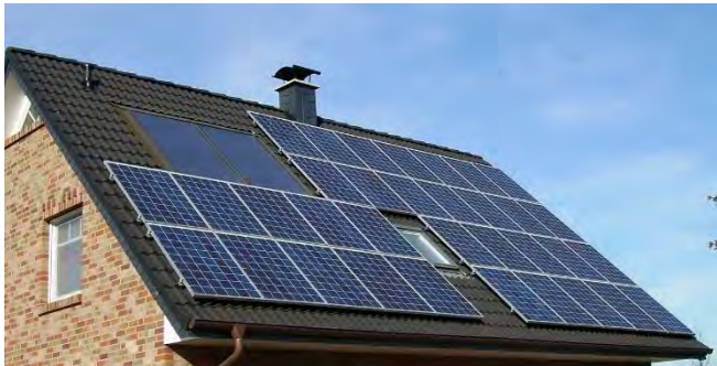
Figure 21: Rooftop Mounted Solar Panels
