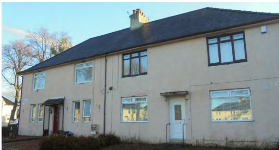
Figure 18: Mismatching window panes and the removal of mullions detract from the original character of these properties (EAC DP&R).
