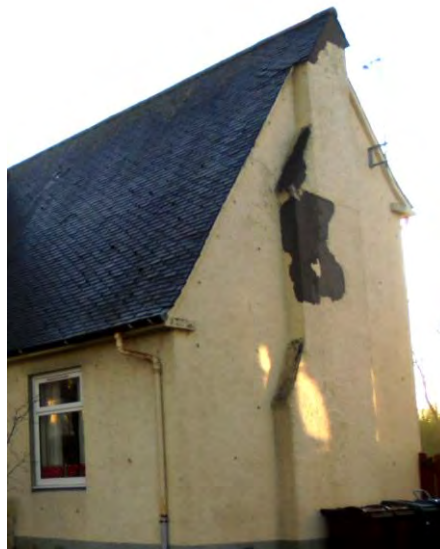
Figure 11: removed chimney stack and wall repairs made with cement mortar (EAC DP&R).
